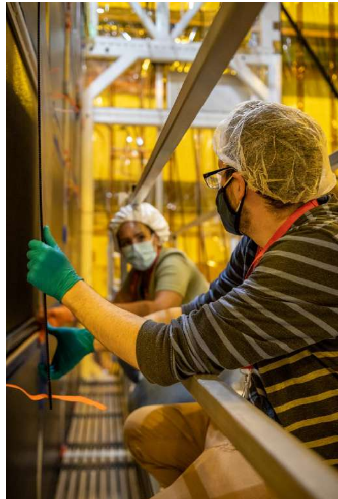
Cathode installation at SBND in the D0 building. Pictured: Mônica Nunes, Vincent Basque. Photo: Ryan Postel
