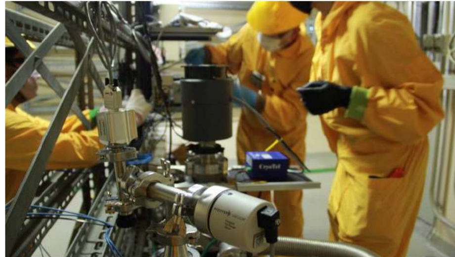
Installing the detectors at Atucha 2 (Image: Nucleoelectrica Argentina)
